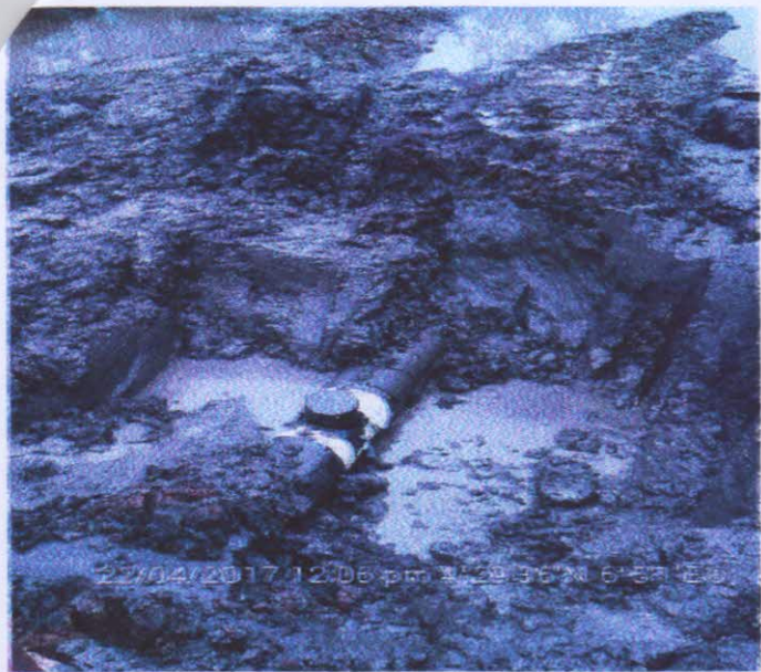
Figure 1: Cut-off Nipple on the pipeline.
